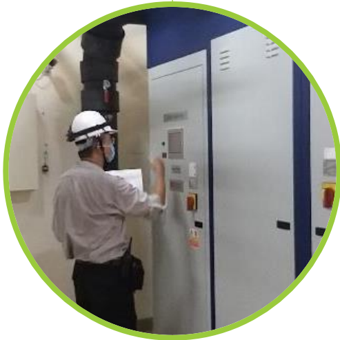
Operation of N2 gas purification equipment
